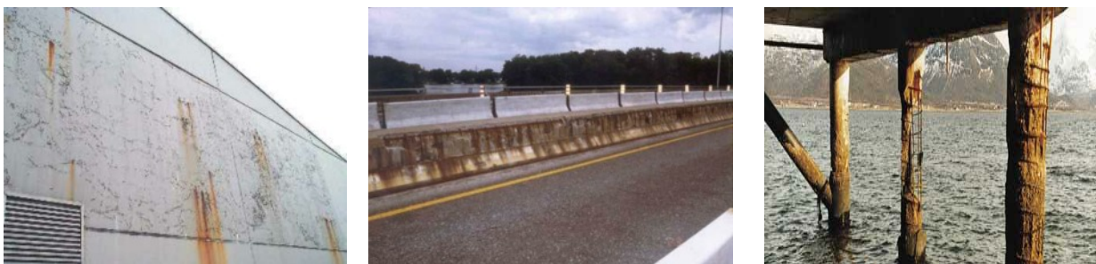
Figure 7.1: Examples of chloride induced corrosion
