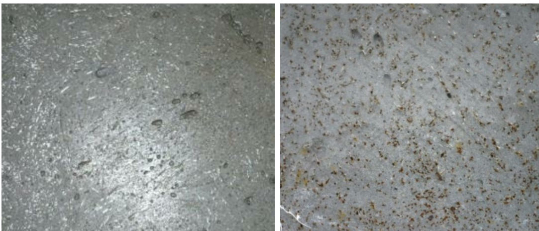
Figure 8.3: Surface of steel-fibred concrete with 0,3% ConcreCem at 7 cycles of freeze-thaw testing and after 14 cycles.
