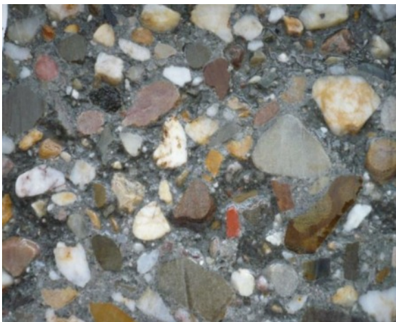
Figure 8.3: Surface of 205 days old concrete without ConcreCem after 14 cycles of Freeze-thawing
