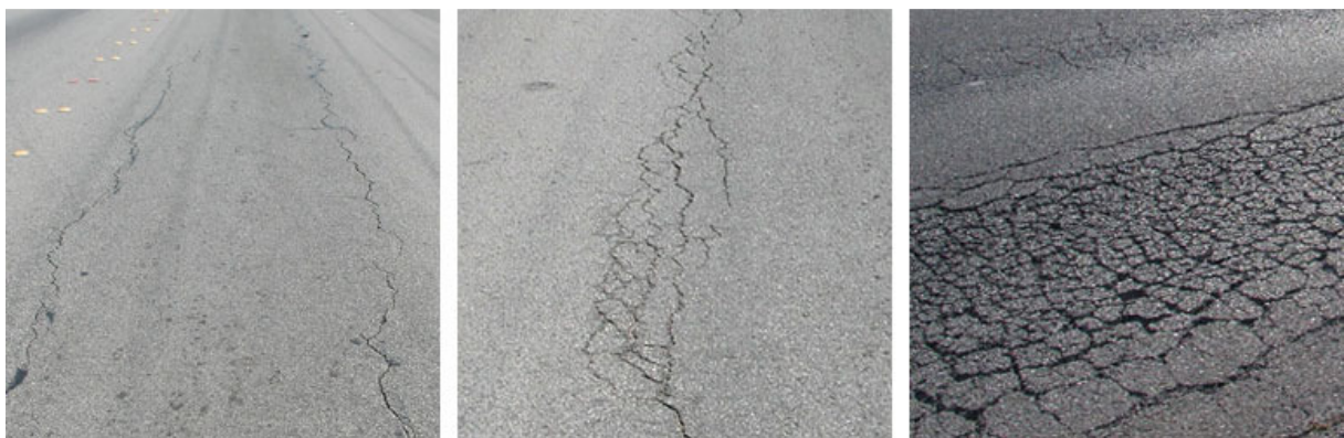
Figure 5.39 Fatigue Cracks in asphalt.
