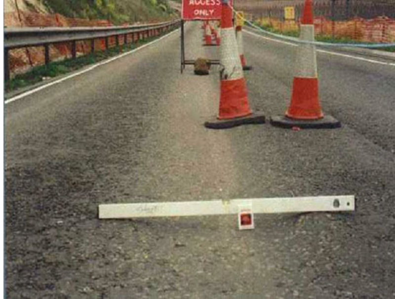
Figure 5.38 Deformation in unbound foundation.
