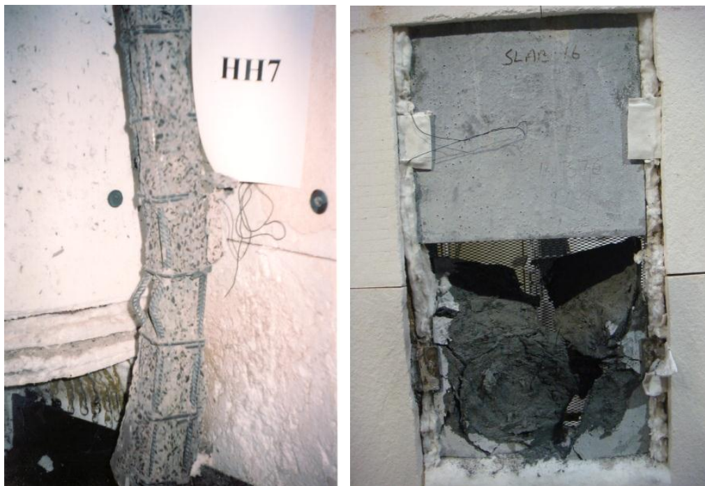
Figure 3. Destructive effect of explosive spalling.
